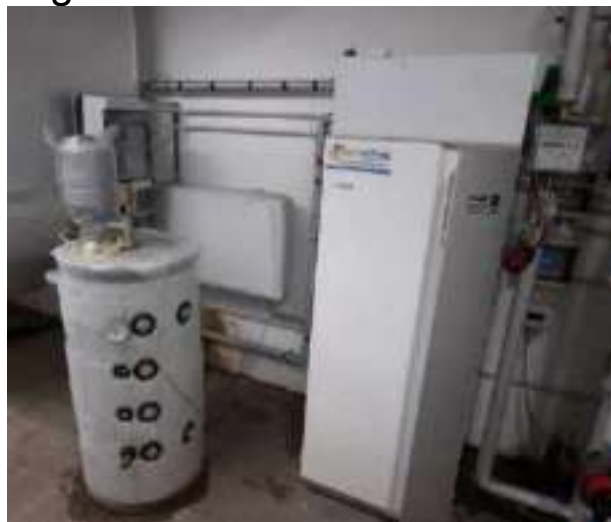
Figure 2: NIBE heat pump of the center with a buffer tank and fan coil
