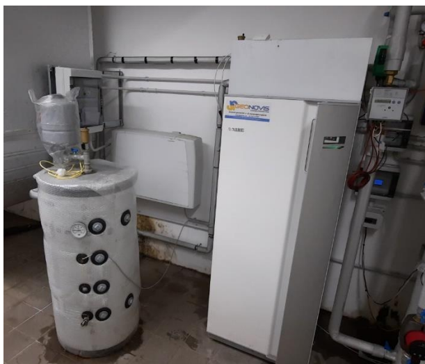
Figure 2: NIBE heat pump of the center with a buffer tank and fan coil
